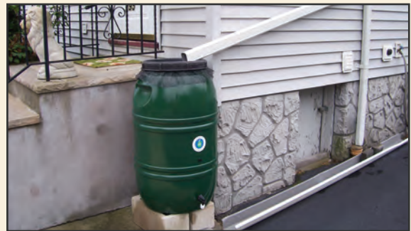
Rain Barrel and Disconnected Downspout City of Paterson
