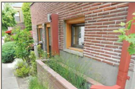
Contained stormwater planter with disconnected downspout Photo courtesy of US EPA
