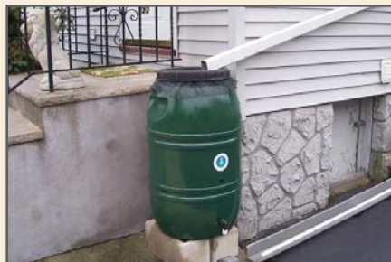
Rain Barrel, Paterson, NJ Photo courtesy of Passaic County Planning Department
