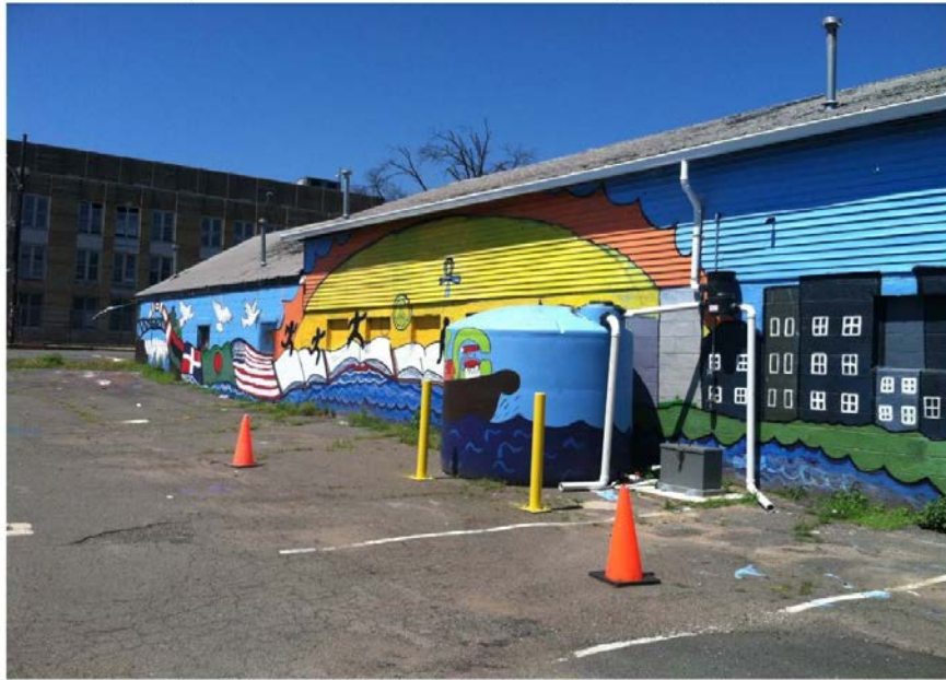
Figure 2: PS5 Cistern; Source: Paterson Public School #5 Green Infrastructure Information Sheet, 2015
