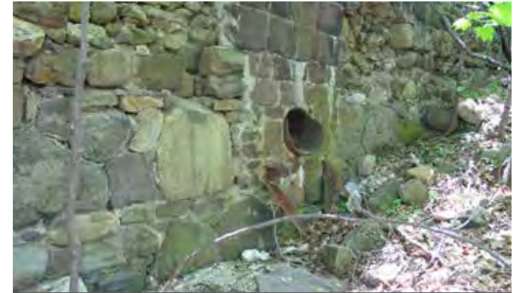
Opportunity: Middle Reservoir ruins offer the opportunity to tell the story of how the river, and local topography shaped by the river, enabled the Passaic Water Company to provide water to the growing nineteenth century city of Paterson. (photo: G. Archimede)
