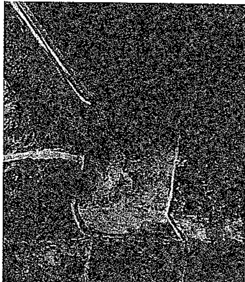
15. A4.6 ST12: Grey cementitious stone patch inappropriate, causing adjacent stone to fail.
