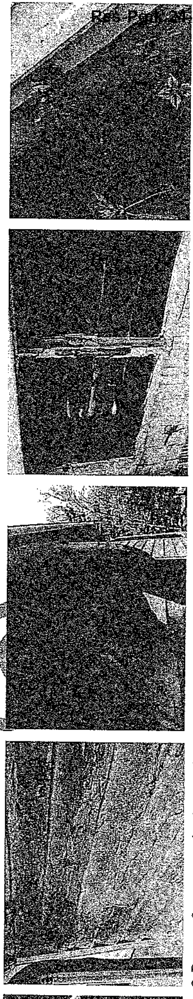
2. Poor surface preparation has resulted in uneven heavy paint build up, which causes water to overflow resulting in blocked gutters and downspouts. 3. Blocked gutters and downspouts cause water to overflow resulting in cracked, dried out, cracked, and cracked glazing putty surrounding the glass panes. 4. The glazing putty surrounding the glass panes has dried out, cracked, and cracked. 5. Excessive plant growth adjacent to the building can cause water saturation.
