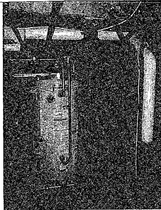
Fig. P-7- Water Heater
