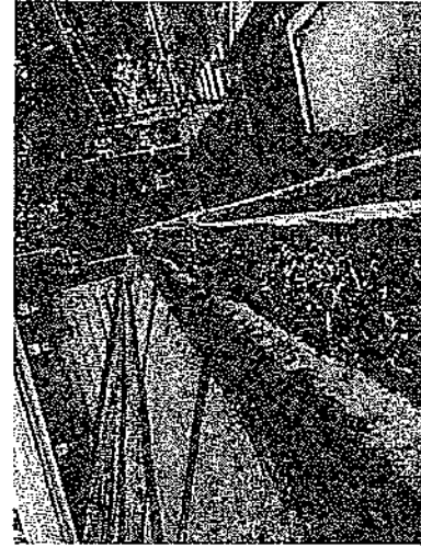
9. The half-round gutter on the (East) side of Roof RF03. The gutter
