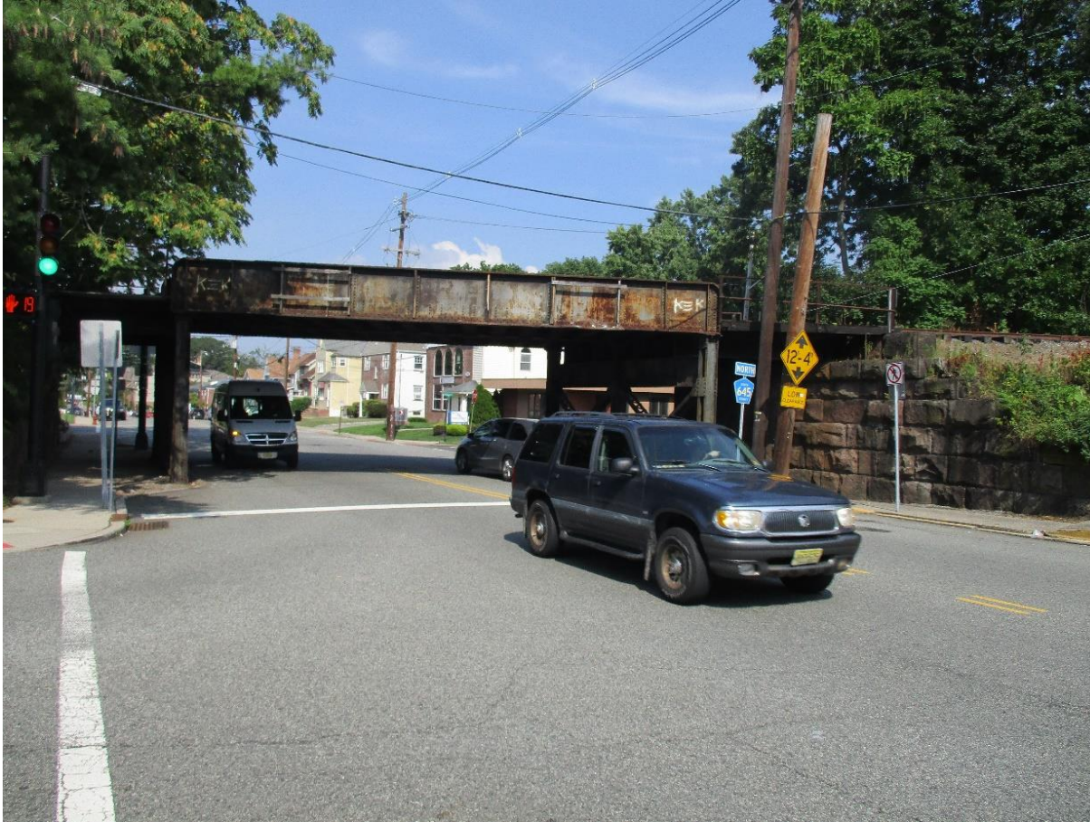
12'4" Substandard Vertical Clearances (Franklin Avenue, Nutley)
