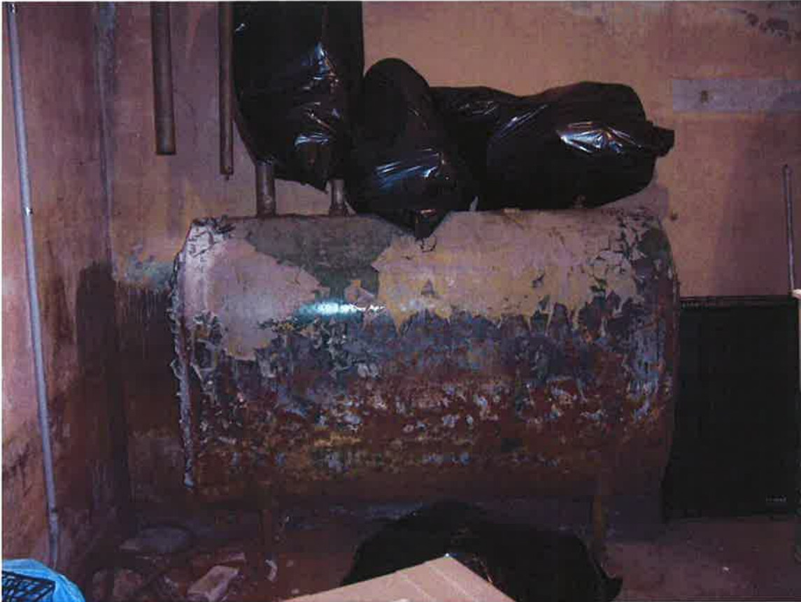
Photograph 11: Out-of-use AST and disconnected fill port and vent pipe located in the basement of the animal control building.
