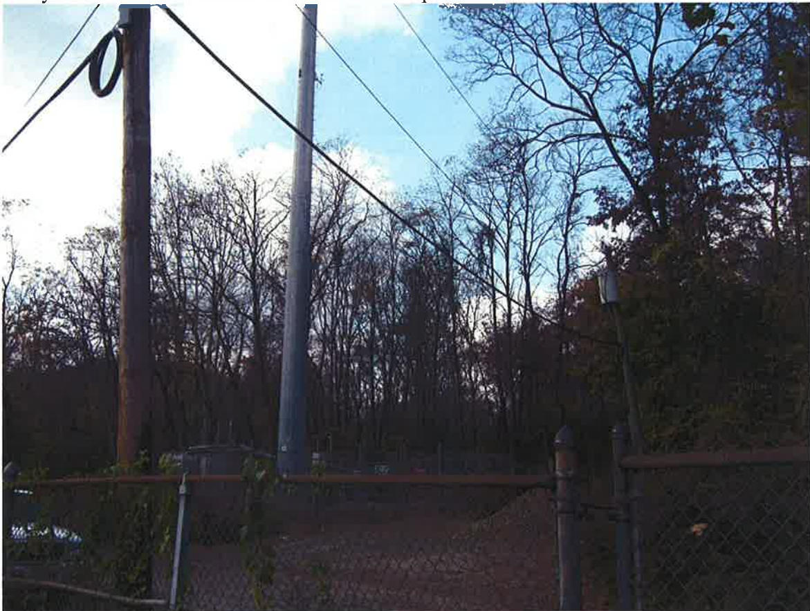
Photograph 20: View of the cellular tower and a pole-mounted transformer located to the west of the on-site structures, facing southwest.
