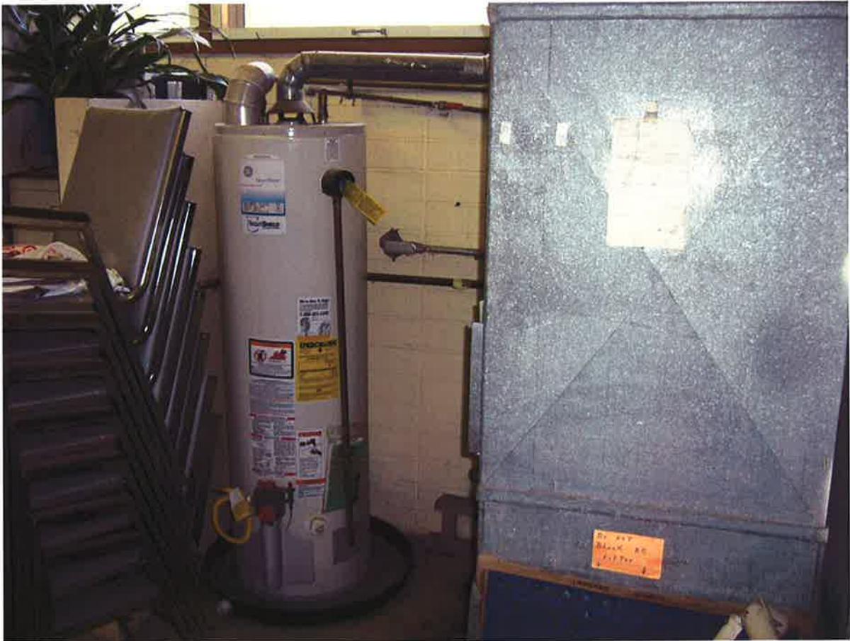
Photograph 3: Hot water heater located in the dog building.
