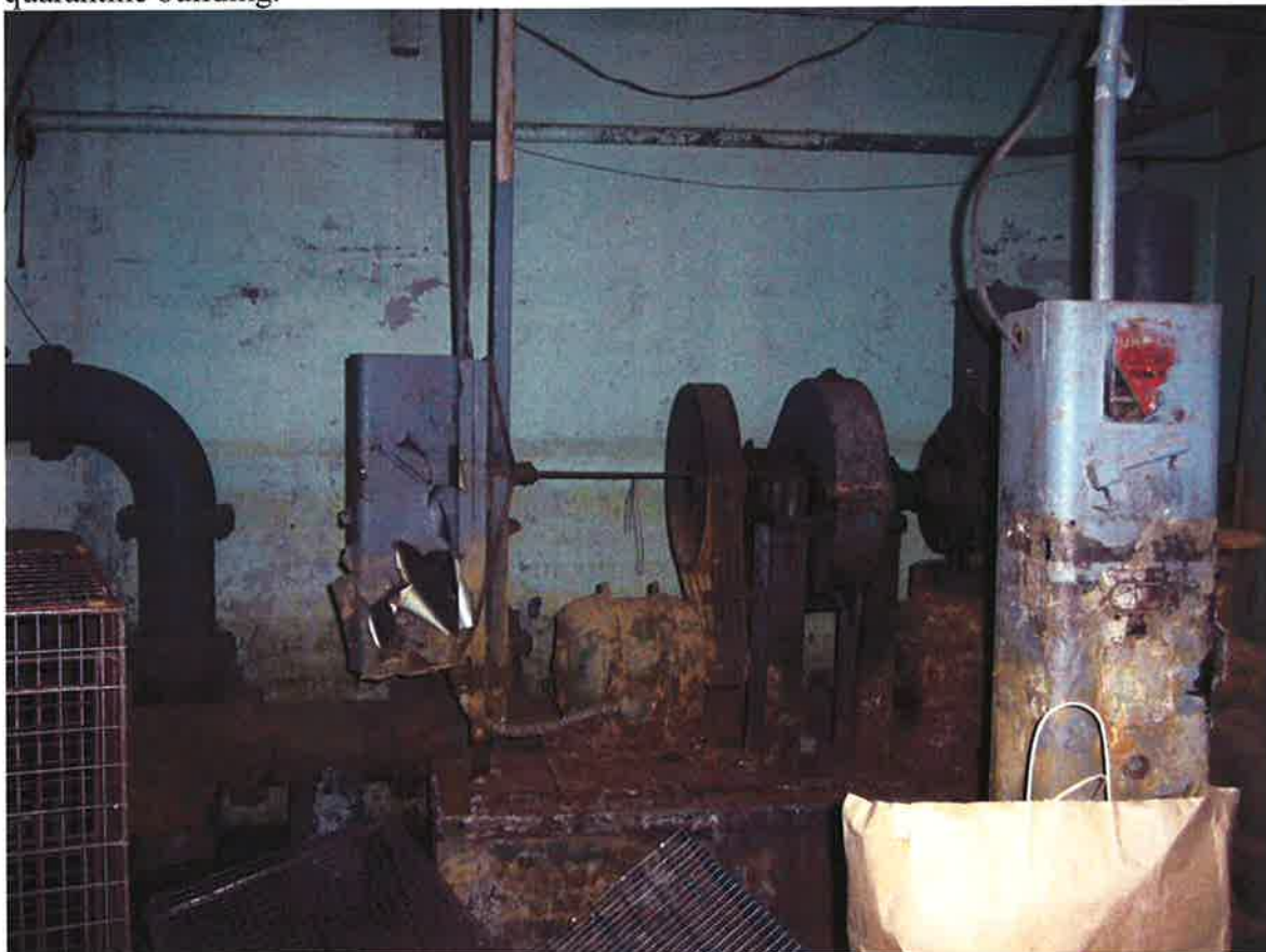
Photograph 8: Old piping and machinery observed in the basement of the animal control building.
