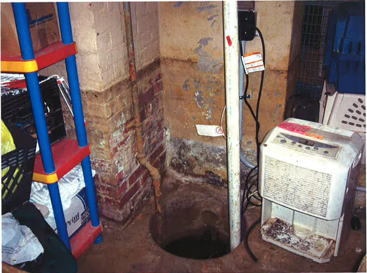
Photograph 9: The sump pump observed in the basement of the animal control building.
