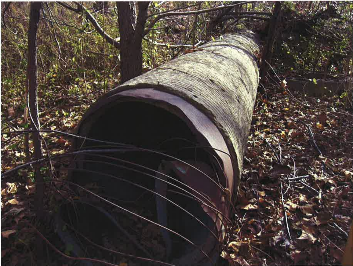
Photograph 19: Large piping located in the wooded portion of the subject property, most likely associated with former sewer treatment operations.
