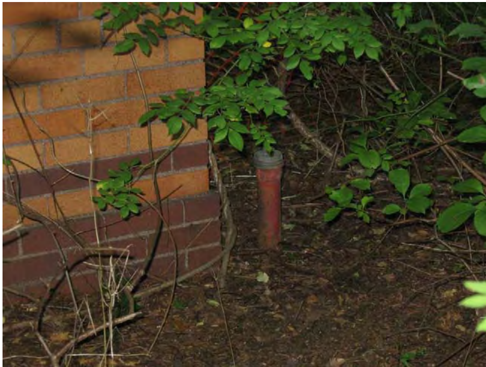
Fill Port for Fuel Oil UST
