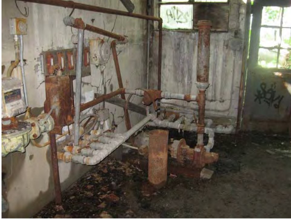
UST Piping Entering Solvent Room
